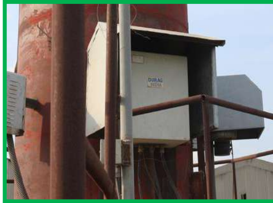
Cement Mill-2 Opacity meter
