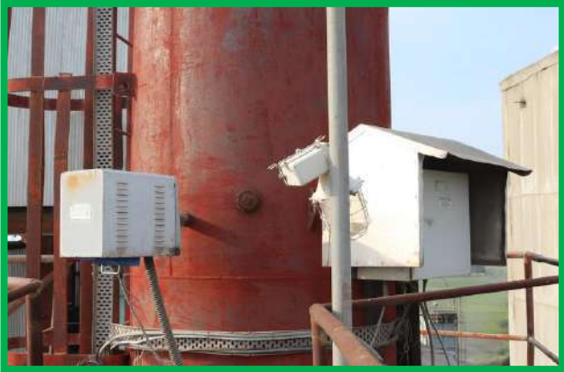
Cement mill- 1 Opacity Meter
