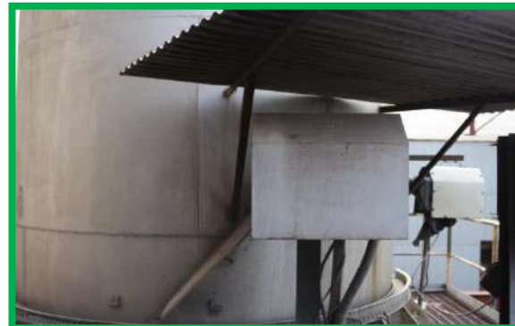
Coal Mill Opacity Meter
