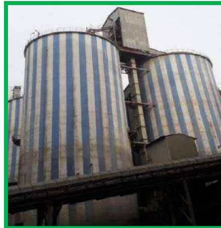
Cement Silo: 4×5000 Tonne
