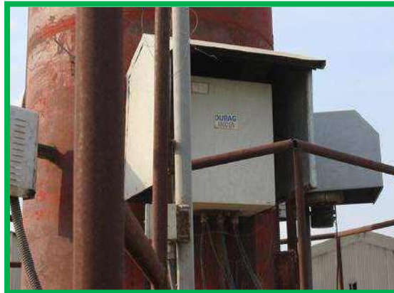
Cement Mill-2 Opacity meter
