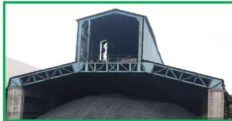
Additives Storage Shed: 15000 Tonne
