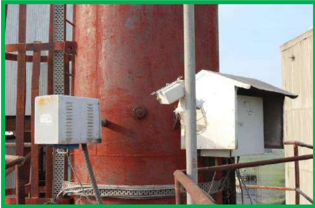
Cement mill- 1 Opacity Meter
