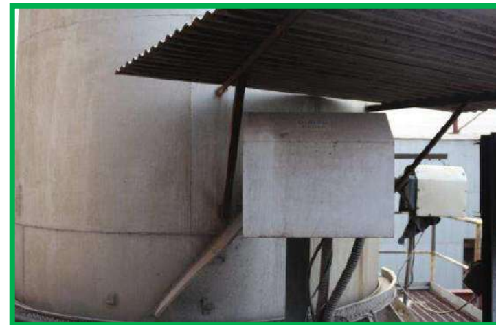
Coal Mill Opacity Meter
