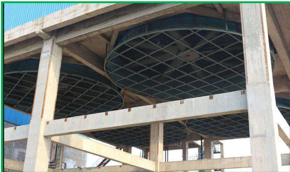
Air Cooled Condensers installed at Captive Power Plant
