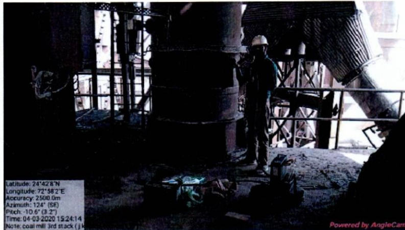
Coal Mill 3 [24°42'8"N 72°58'2"E]
