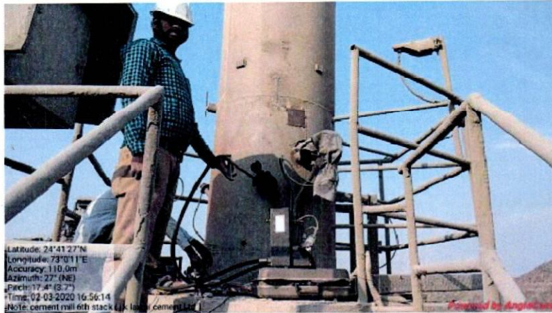
Cement Mill No.6 [24*41'27"N 73*0'11"E]
