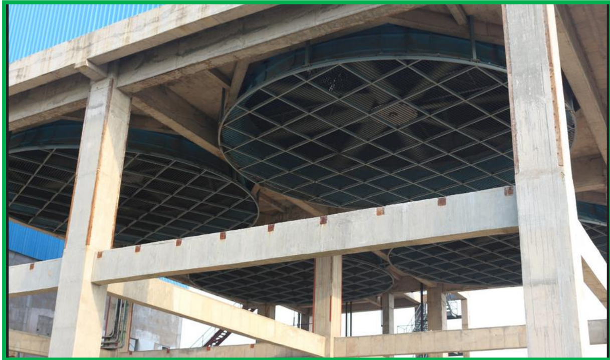
Air Cooled Condensers installed at Captive Power Plant
