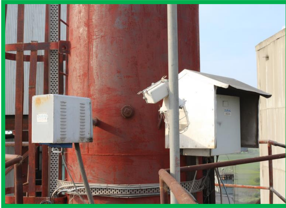
Cement mill- 1 Opacity Meter
