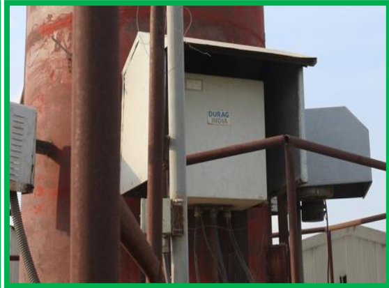
Cement Mill-2 Opacity meter
