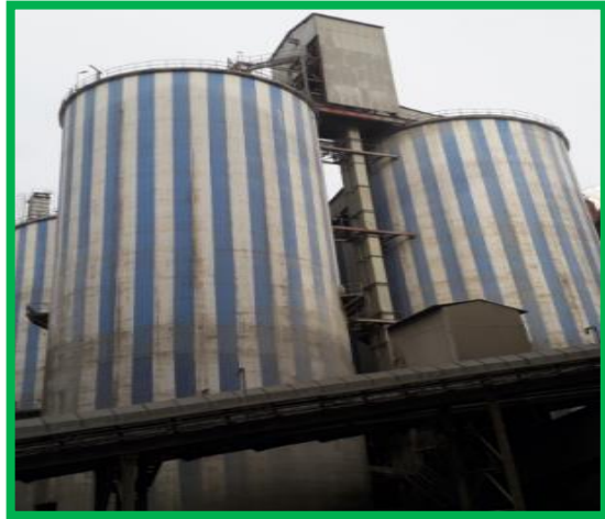
Cement Silo: 4×5000 Tonne
