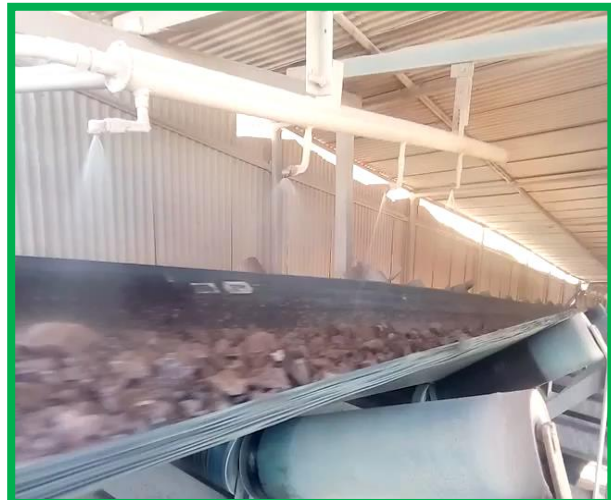
Water Sprinkling Systems in conveyor belts
