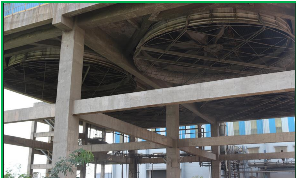
Air Cooled Condenser installed at Waste Heat Recovery
