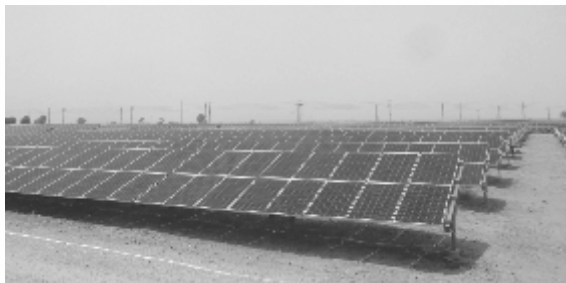
6 MW Solar Power Plant at Phalodi, Rajasthan
