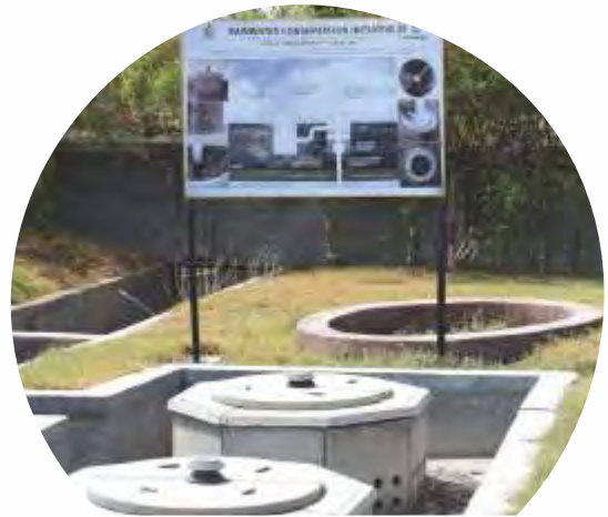
RAINWATER HARVESTING AT KALOL PLANT
